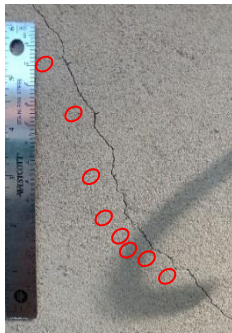
Figure 4: Locations of crack width measurement along the crack
