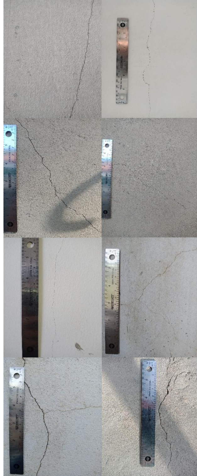
Figure 3: Photographs of cracks considered
