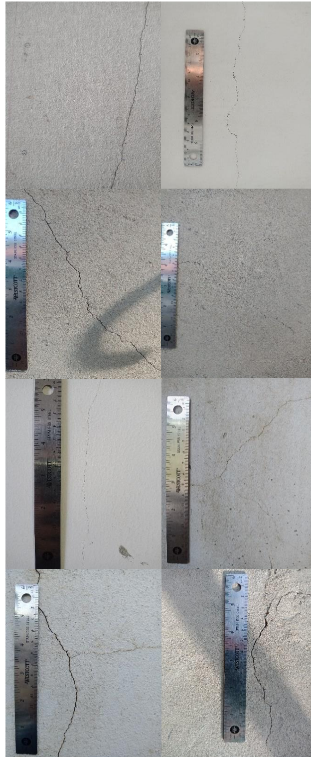
Figure 3: Photographs of cracks considered
